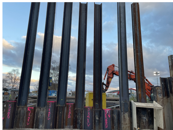
(b) Spontinstallation, del 2.
